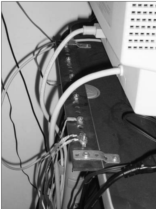
Figure 13-10: A copper ground bus installed in my shack.
